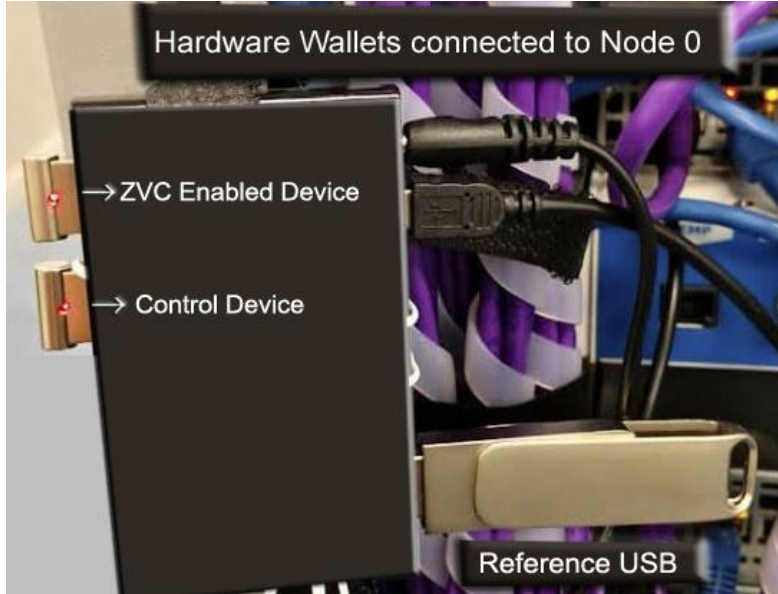
Mounted ZVC device & Control device
